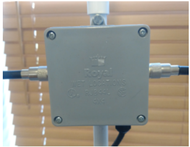
Outdoor Utility box.
