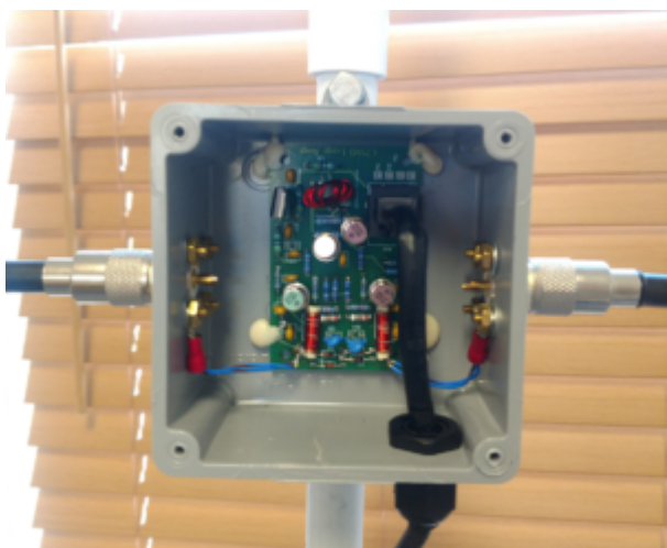
LNA mounted in box
